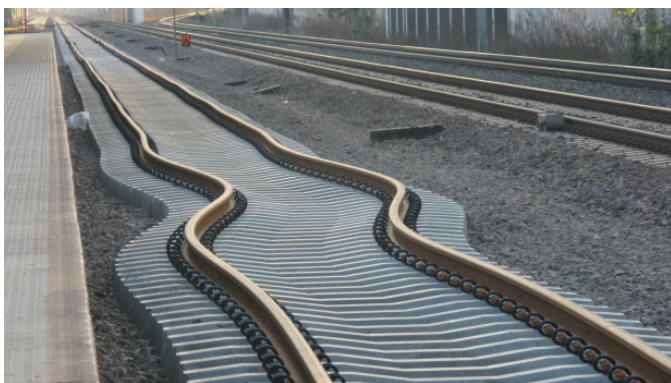
Fig. 1. Contactless track buckling [8]
