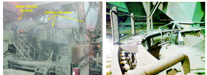
Fig. 11. Water-Cooled Channel Containing the Camera Services (Aldwarke ‘N’Furnace)
